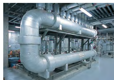
This heat exchange system cools our injection molding equipment with heat from an electrical generator.
