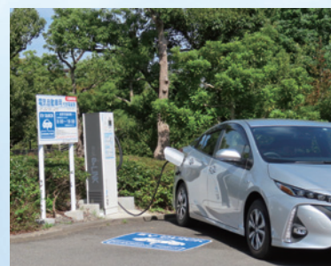
eLINK installed at a public facility
