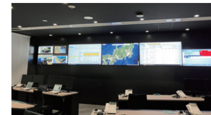
The call center in our Tokyo Service Center
