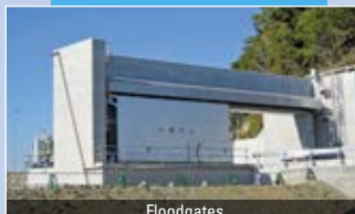
Floodgates Cable carriers
