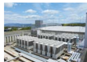
High efficiency chiller (Kyotanabe Plant)
