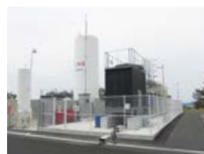
Heat supply system through gas power generation (Okayama Plant)
